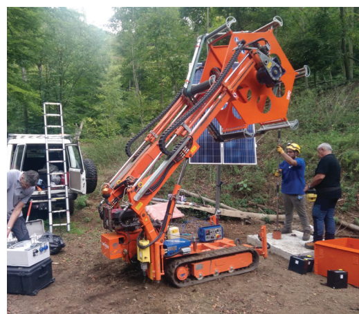
Installation of a DMS multiparametric inclinometer by CSG at the Čeřeniřtř landslide site (CZ)
